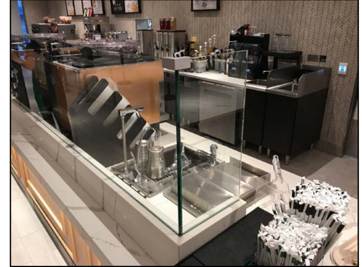
Sneeze Guard Installed at Starbucks
